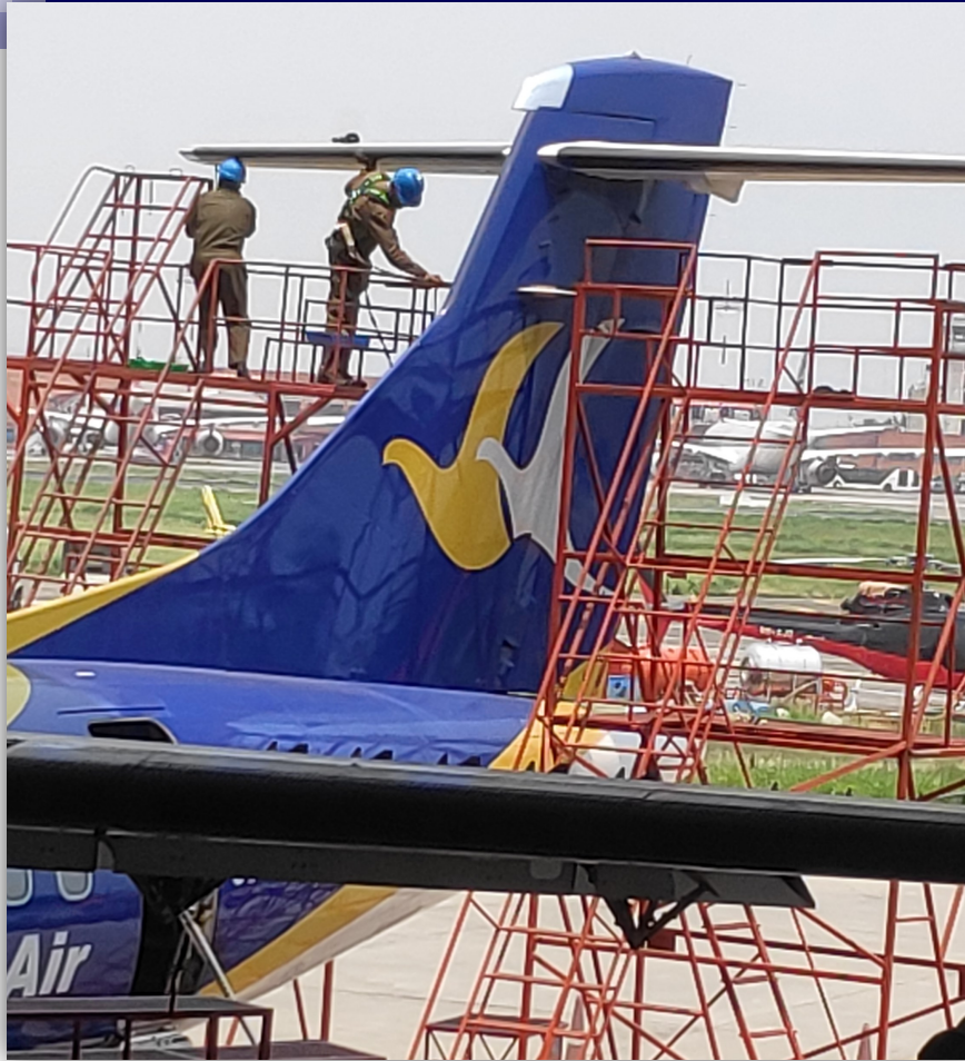
Use of PPE while working from heights
